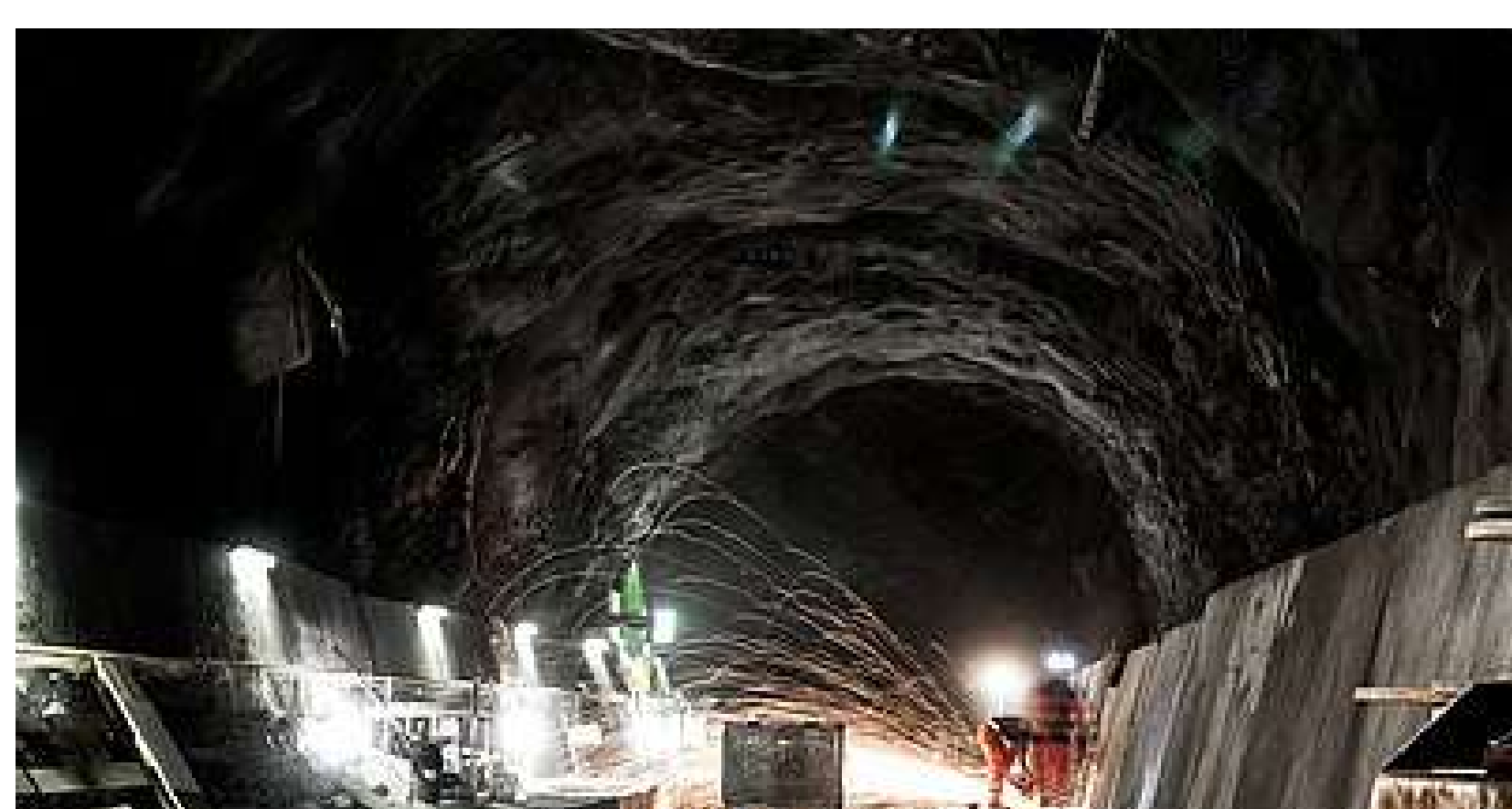
Underground Future Lab – Nationally significant innovation center leading the digitalization of tunnels
